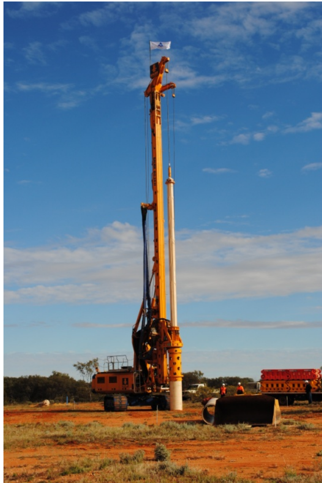
“Big Bertha” BG 28H rig on site at Arafura’s Nolans Rare Earths Project, Northern Territory
